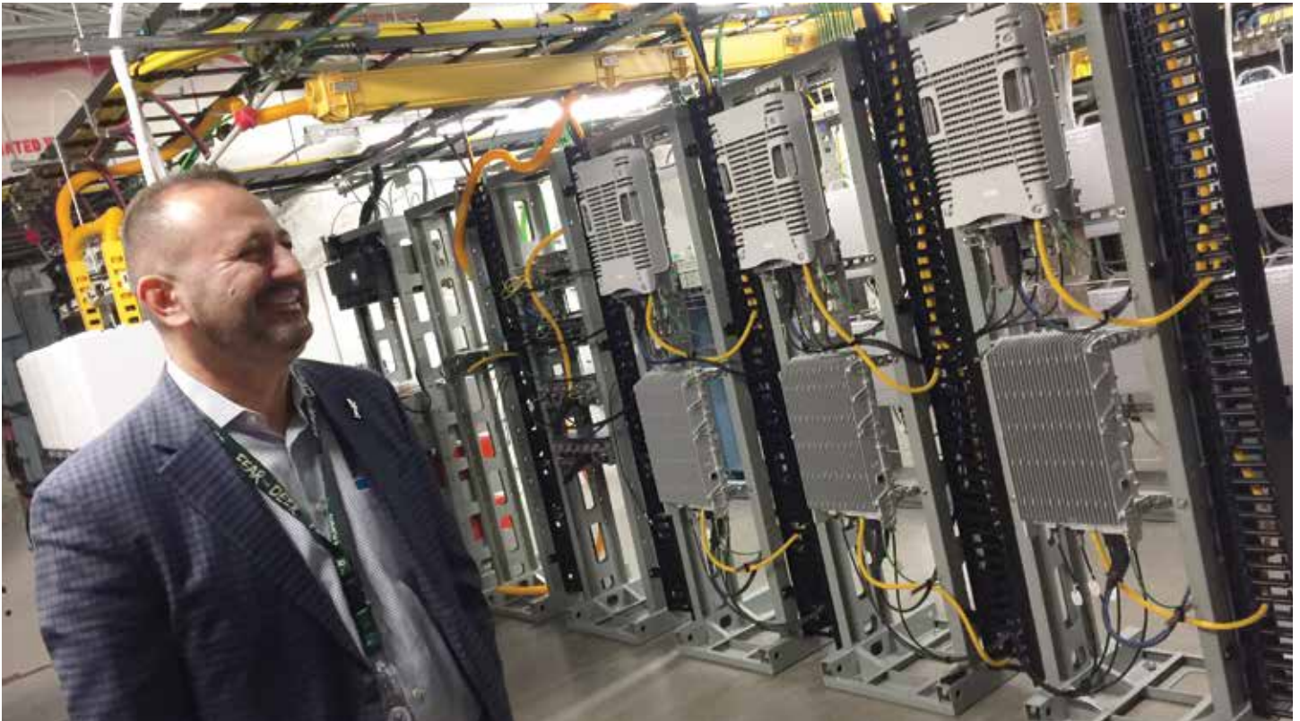
FACING PAGE: FISERV FORUM'S ENTRYWAY GLOWS AT NIGHT. THIS PAGE: THE BUCKS' ROBERT CORDOVA IN THE DAS HEADEND ROOM. CREDIT ALL PHOTOS: PAUL KAPUSTKA, MSR
